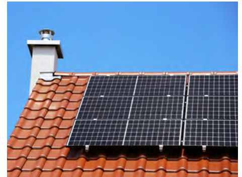
Figure 2 – Solar PV systems may be installed with electric heat pump water heaters serving high-rise residential dwelling units or hotel/motel guest rooms as a new prescriptive water heating compliance option in the 2019 Energy Code
