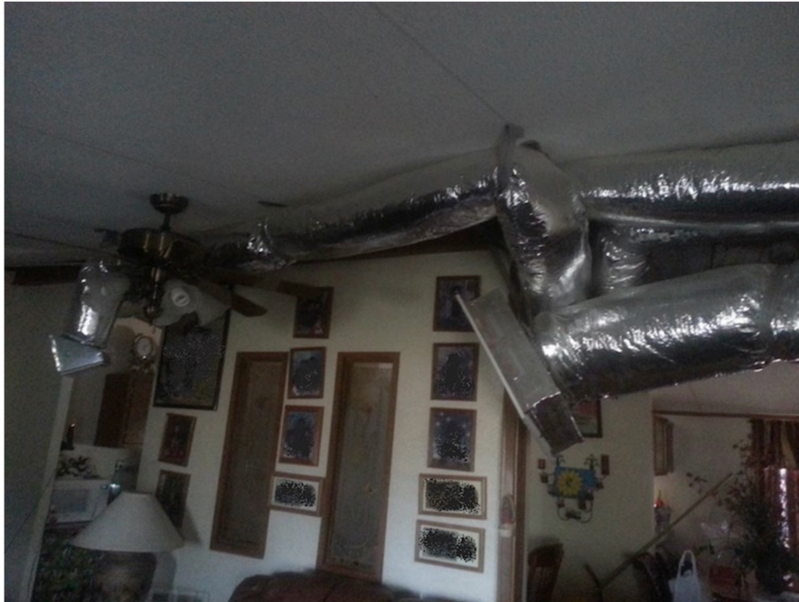
A bad way to get ducts inside the conditioned space [Source: HVAC Hacks & Other Screwups]
